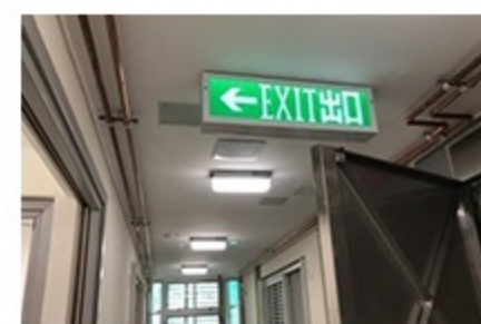
LED Exit Sign
