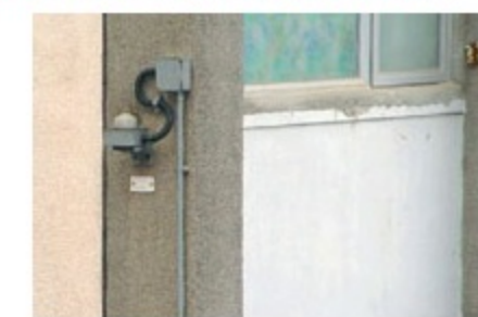
Photocell sensor controls for lights
